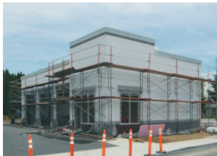
Jiffy Lube, Wilsonville, Oregon. This three-bay facility was constructed for Lube Development LLC.
