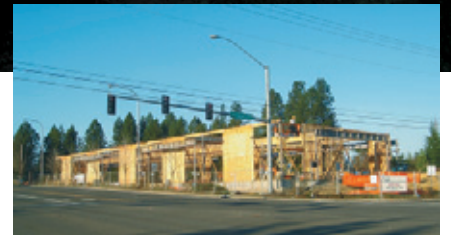
Baseline Station Retail Building, Hillsboro, Oregon. Owned and developed by Baseline Station LLC, this 12,000-square-foot building was about 50% pre-leased when construction began last fall. Designed by Robert Evenson Associates, it will provide much needed space in the rapidly developing light rail transit corridor.
