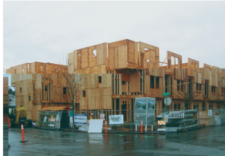
Building One of the Belmont Townhomes awaits roof trusses as a rainy winter slows projects all over town. This 28-unit condominium project will be completed this summer.
