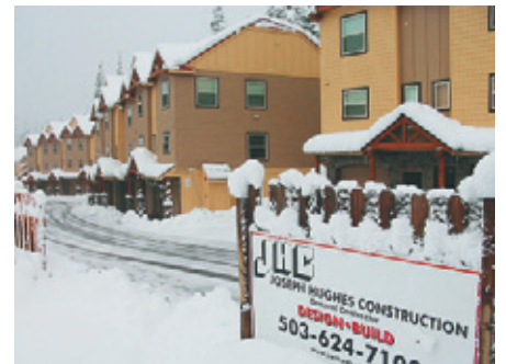
On Mount Hood at Government Camp JHC crews completed the first 151 units of the Collins Lake Resort Condominium project this spring. Snow was a critical challenge during the three-year job.
