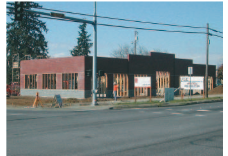
The Sirrah Office Building is a 4,800-square-foot office structure designed by the JHC team in conjunction with David Bissett and Associates Architects. The owner, Bud Harris, lives next door to the job site and kept close watch on our progress.
