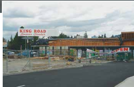
Right: King Road Demo, Milwaukie, Oregon. Demolition crews earned their pay taking down the 120,000-square-foot shopping center.
