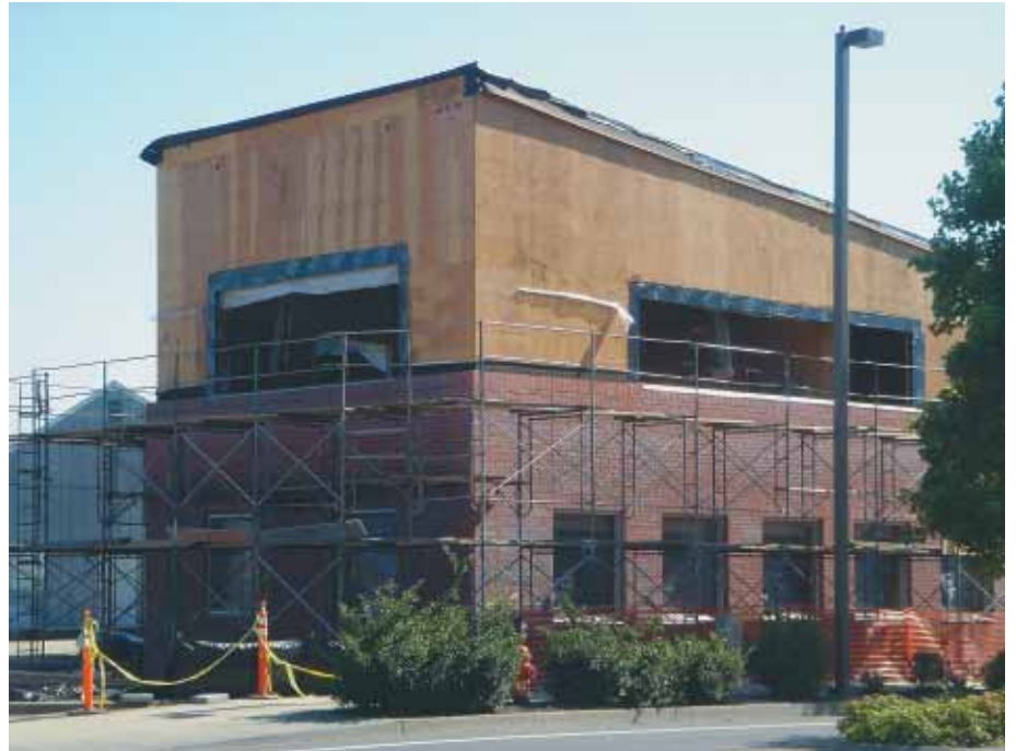
Pioneer Waterproofing Portland, Oregon. This 4,500-square-foot, two-story addition to an occupied office building designed by Soderstrom Architects, P.C., will enhance the expanding operations of Pioneer Waterproofing
