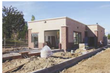
Above: Grease Monkey Quick Lube and Car Wash, developed by Fairfield Auto Company, is a combination oil change/car wash in Battle Ground, Washington.
